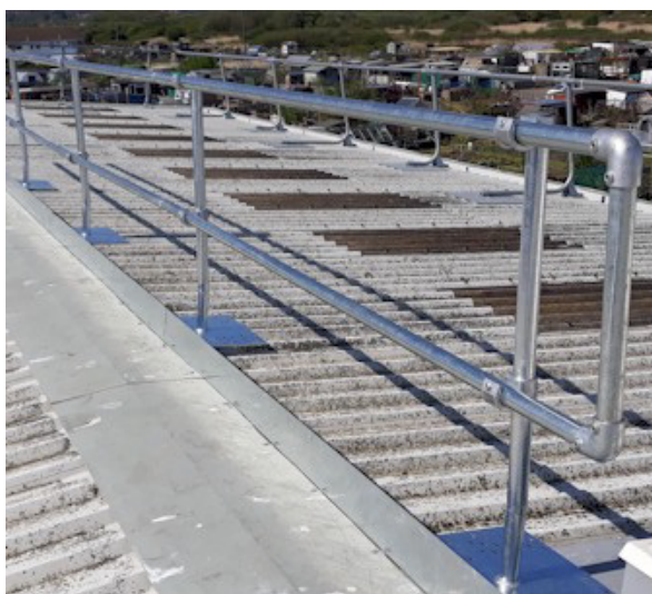
Clad Rail System View of installed system.
