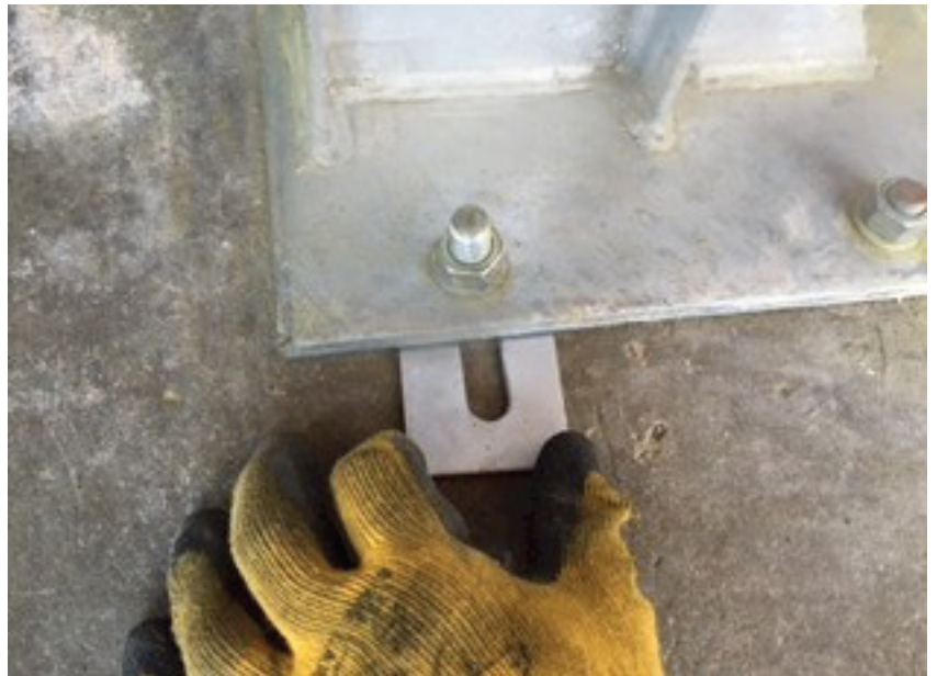
Trouser Shim being inserted under a base plate to align and level the vertical post.
