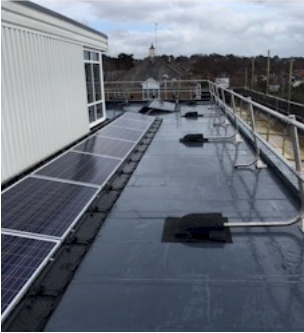
Above Standard FSR Freestand. Stainless Steel Grade 316 Used in a marine environment.
